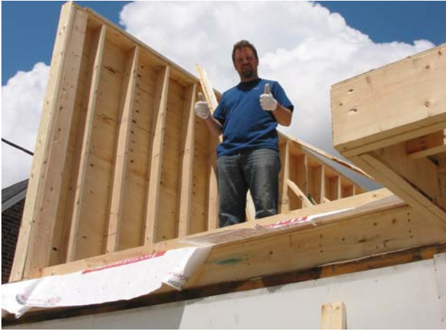
Thumbs up! Stefano takes care of the project from start to finish, personally supervising and inspecting all workmanship.
